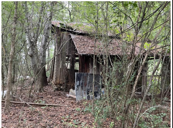
PHOTOGRAPH 8 Dilapidated ancillary/barn structure, northeastern portion of the site.
