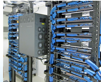
Structured Cabling / IT Systems
