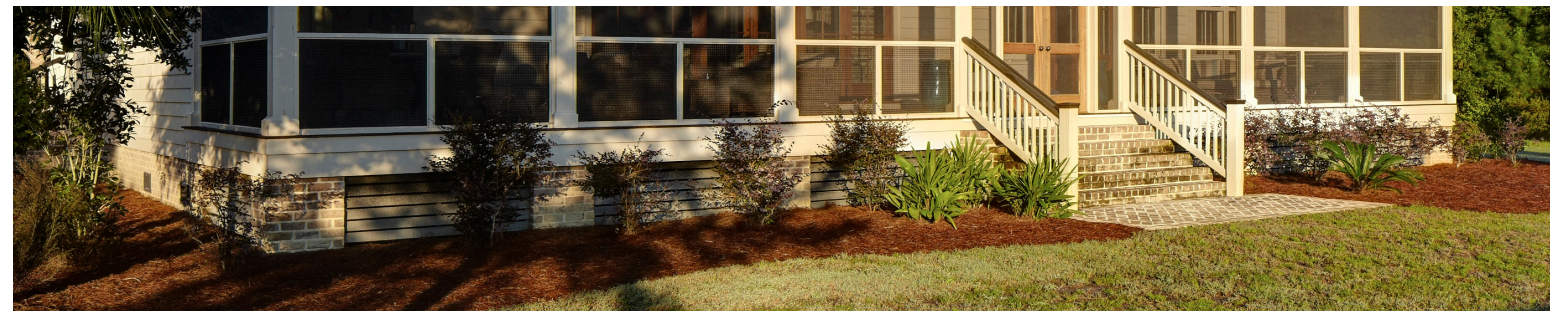
Foundation with louver screening
