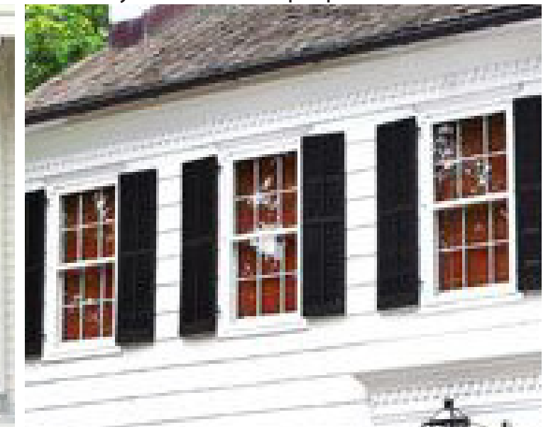
Window trim is the appropriate width
